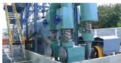
Figure 2: Duo pumps to prevent the system turn off suddenly.
